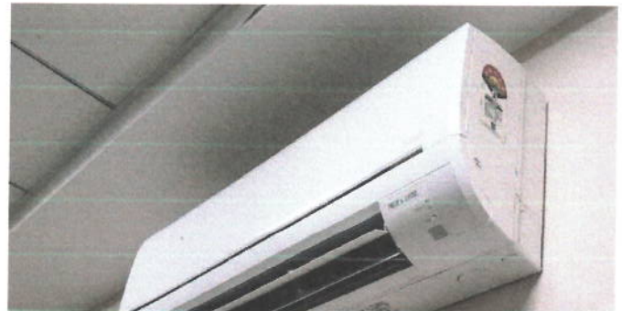
Photo. Air conditioner in server room
