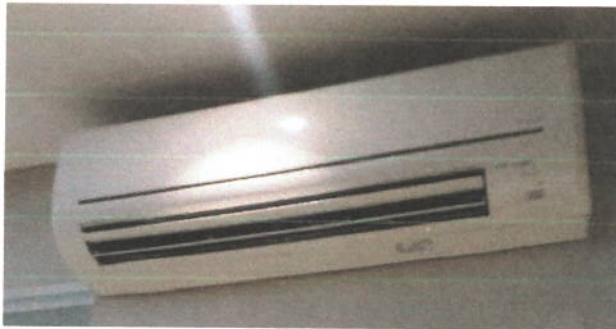
Photo. Air conditioner in board room
