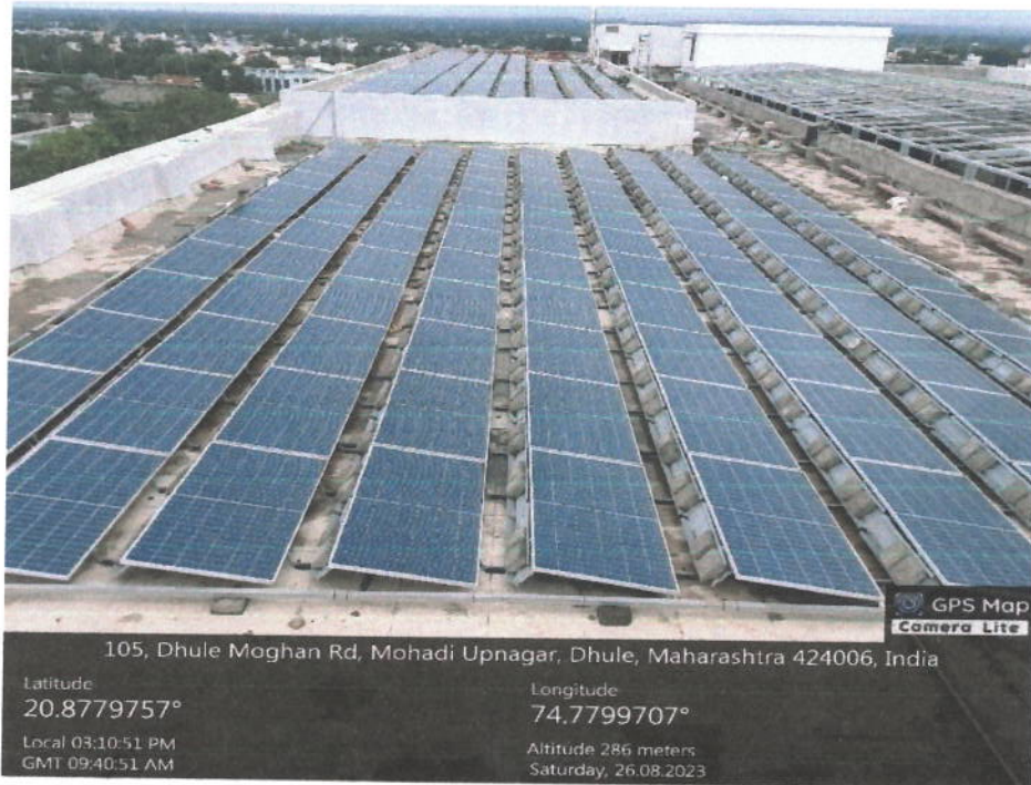
Photo. A view of photovoltaic panels set-up on Institute's Rooftop
